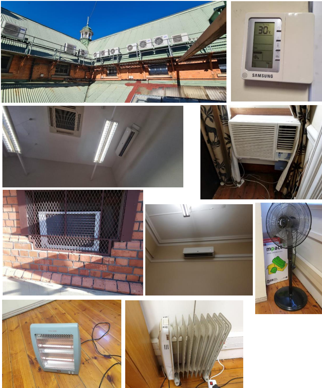
Figure 9: A collection of the split units (wall, through-wall and ceiling cassettes) and personal heating and cooling appliances observed throughout the building.
