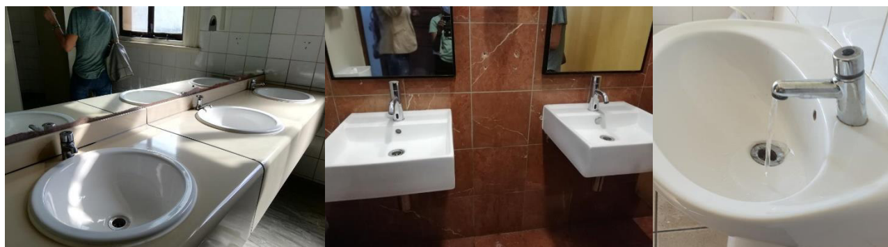
Figure 18: Examples of the various tap fittings and showing the high flow rate of the push taps.
