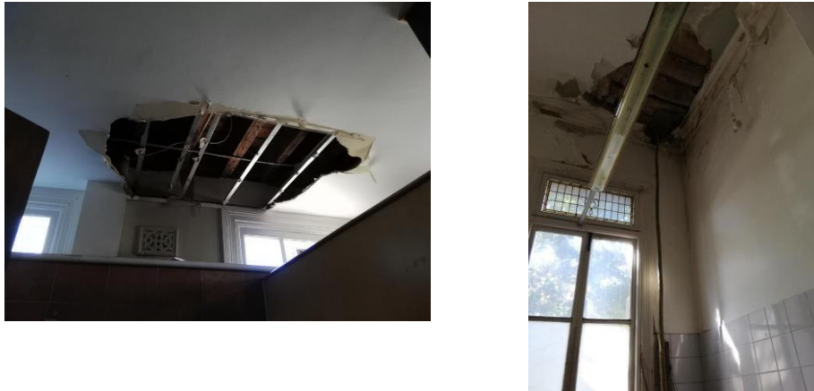
Figure 10: Evidence of ceilings in disrepair in some sections of the building.
