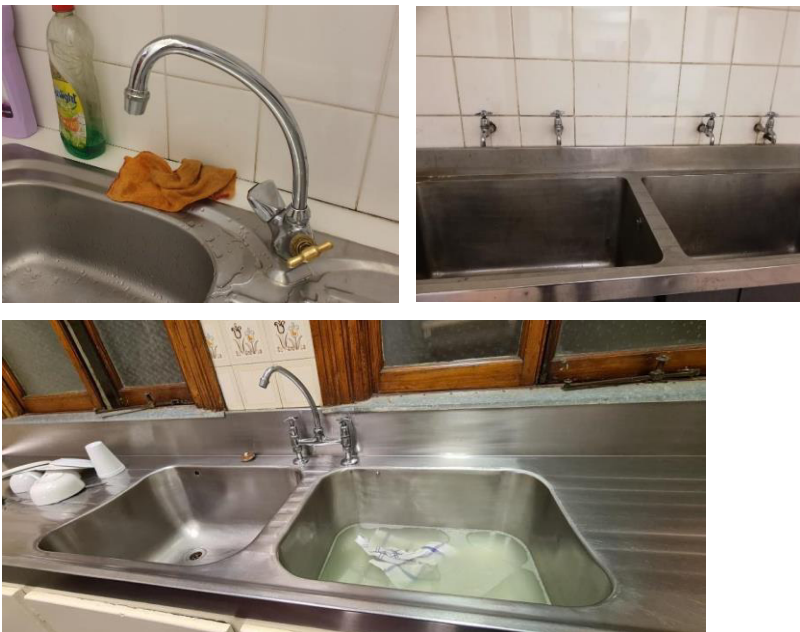
Figure 21: Kitchen tap fittings.
