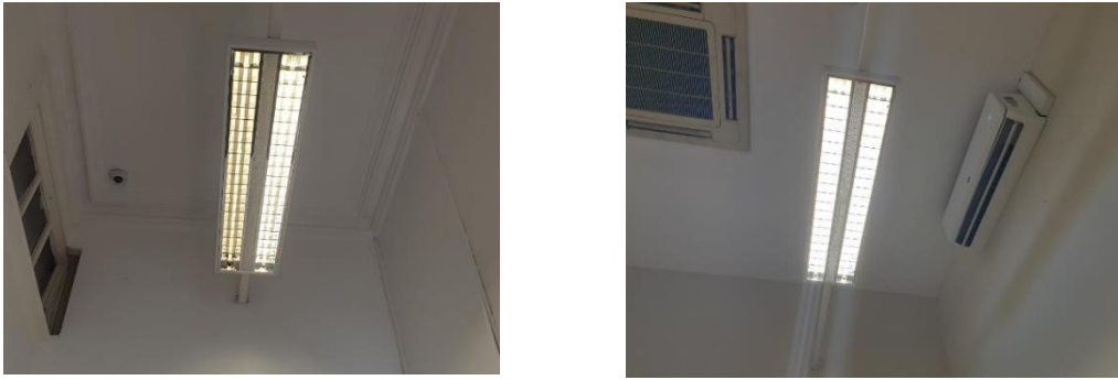
Figure 11: Example of some of the typical light fittings within the building.
